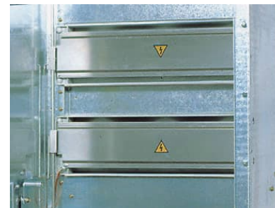
Segregating shutters with metal partitions
